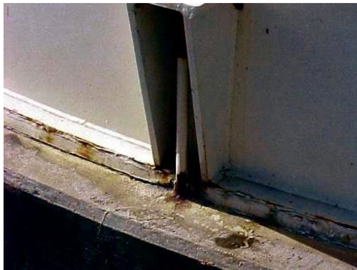
Figure 21—Anchor Bolt with Suspected Corrosion
