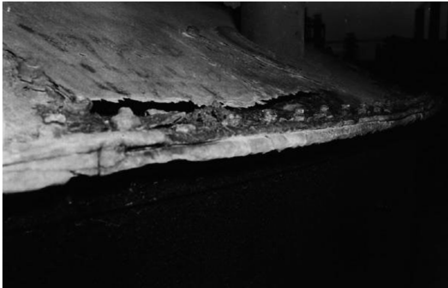
Figure 31—Example of Severe Corrosion of Tank Roof
