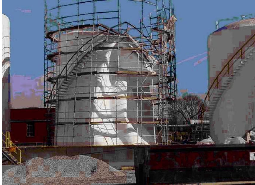
Figure 29—Tank Failure Caused by Inadequate/Obstructed Vacuum Venting
