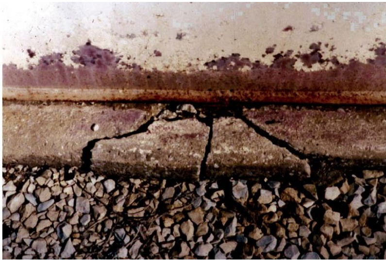
Figure 20—Failure of Concrete Ringwall
