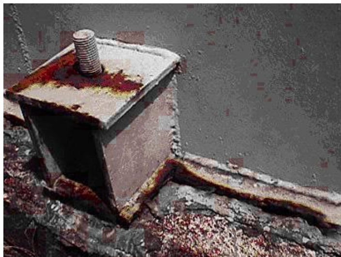
Figure 22—Corrosion of Anchor Bolts
