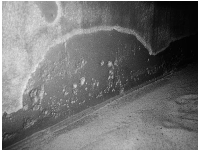
Figure 40—Shell-to-bottom Weld Corrosion
