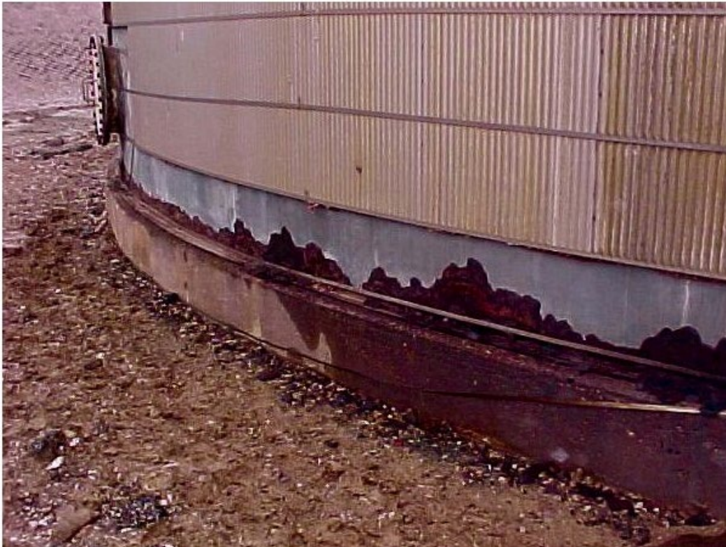
Figure 23—Corrosion Under Insulation
