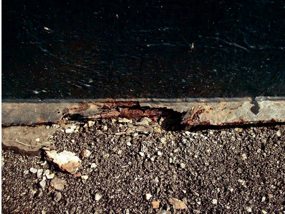
Figure 25—Corrosion (External) at Grade
