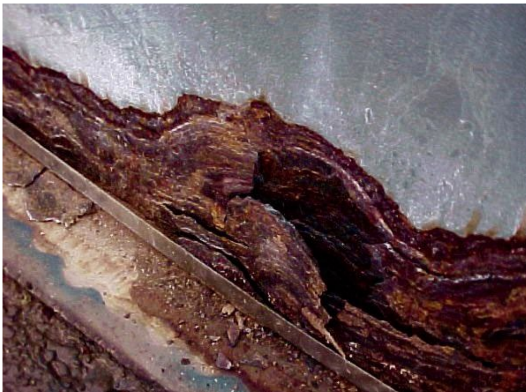
Figure 24—Close-up of Corrosion Under Insulation
