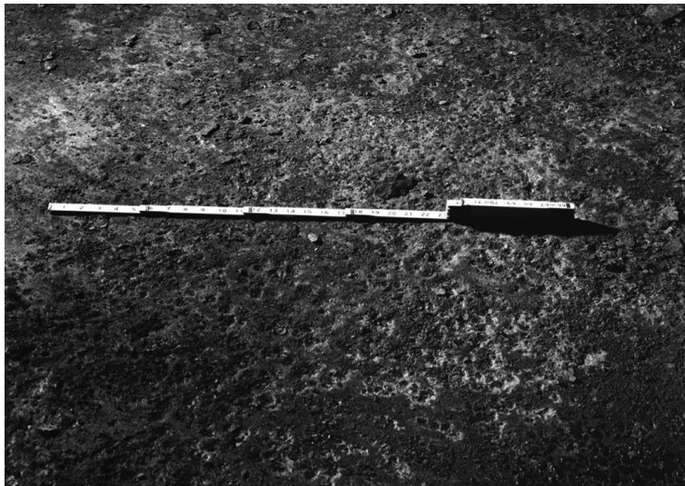
Figure 39—Example of Extensive Corrosion of a Tank Bottom
