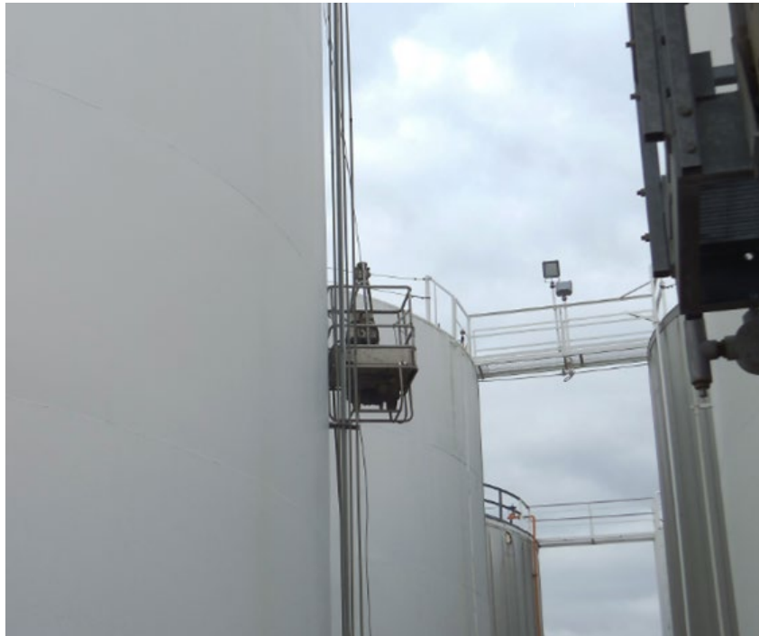
Figure 35—Single-point Suspended Scaffold Used for Inspection and Repairs on Exterior of Tank
