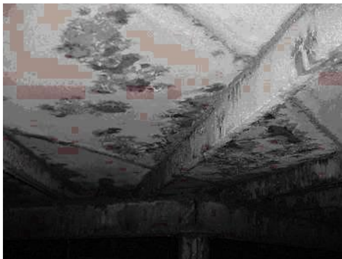
Figure 42—Internal Corrosion on Rafters and Roof Plates
