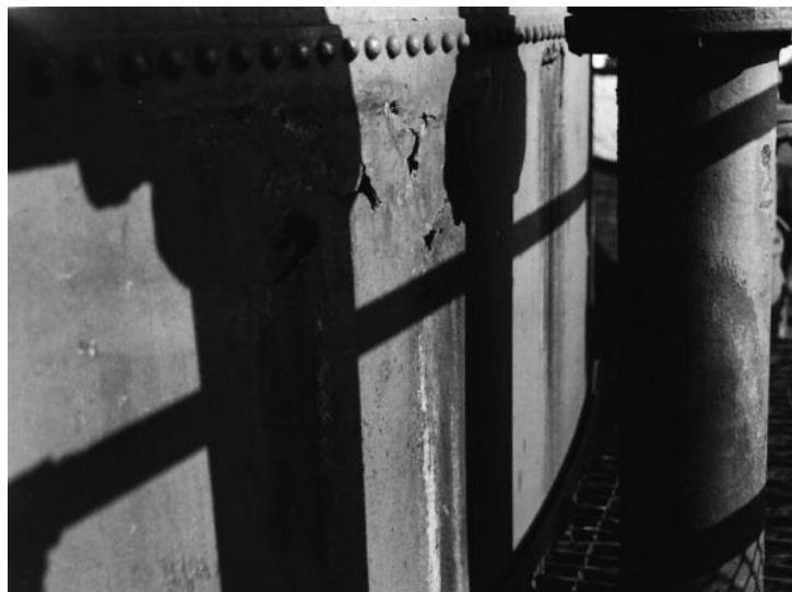
Figure 41—External View of Erosion-corrosion Completely Penetrating a Tank Shell
