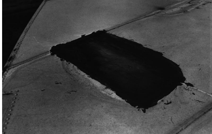
Figure 50—Temporary “Soft Patch” Over Leak in Tank Roof
